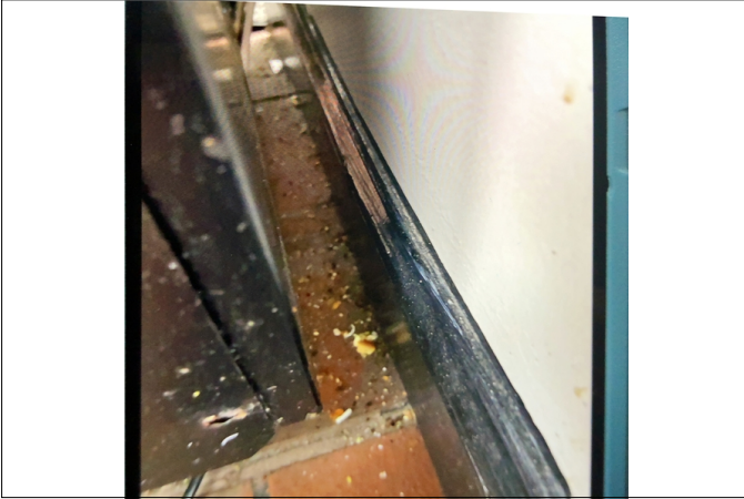
build up between equipment
