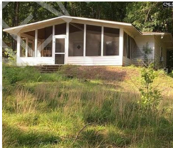
Wood Rot and Termite Damage 142
